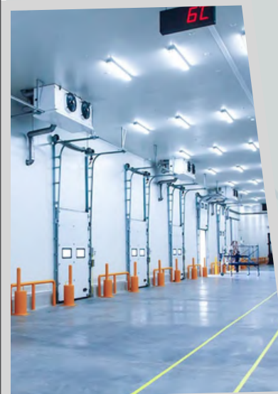
COLD STORAGE & REFRIGERATION
